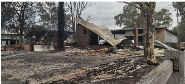
Clifton Creek Primary School devastated in the Black Summer Bushfires, East Victoria
