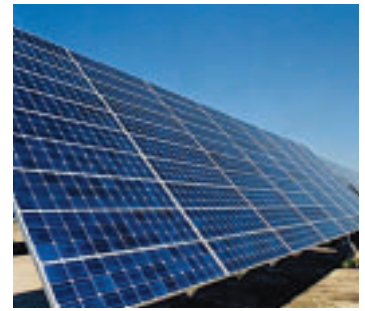
Solar-energy park in Europe.
