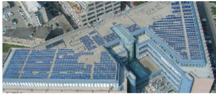
Rooftop solar-power installation using REC solar modules (ScanModule) at the headquarters of UBS Acacias in Geneva.
